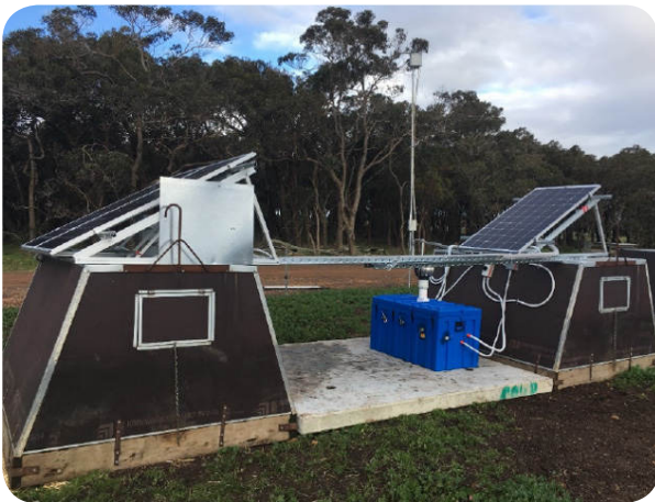
Figure 6. External view of huts showing solar panels, battery storage box and the remote communications tower in the background.
